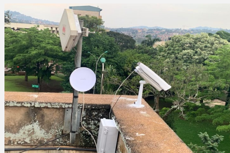
CCTV camera installation complete (side view)
