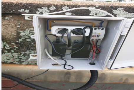
CCTV Camera Control Box
