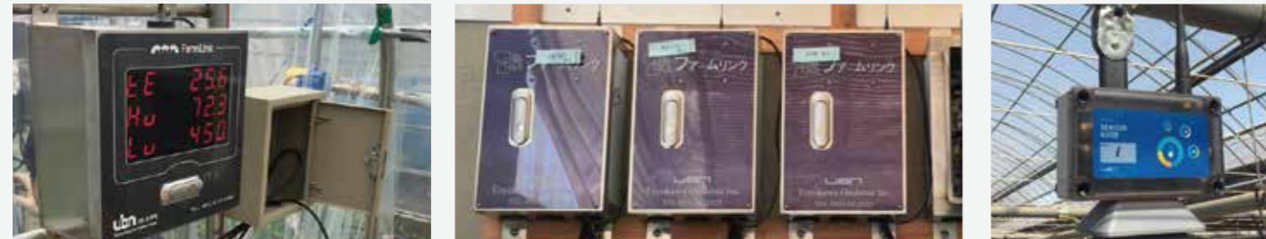
▲ Network Controller ▲ Wireless Actuator Controller ▲ Wireless Sensor Nodes
